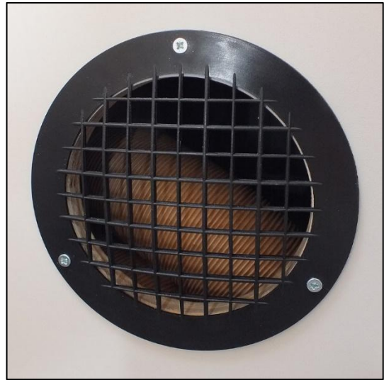
Intake opening for circulating air
